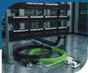
Network Cabling Solutions Ethernet Connectivity in Automation, Data Centre
